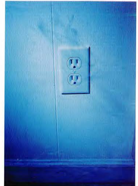
About 15 minutes after Klossner and Greiner fill the Gubbels' garage with theatrical smoke, it streams under the weather-stripped door to the house and billows down the stairway to the basement. Meanwhile, thin wisps trail from an electrical outlet.
