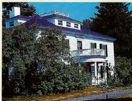
Lovely to look at, Kirkside had rotted sills, a leaky roof and a sunlight-deprived kitchen.
