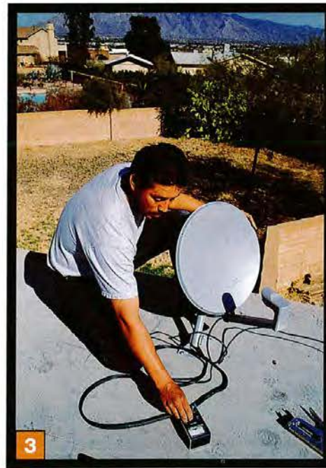
3 Camacho's $150 signal-strength meter enables him to make final, precise adjustments. A less sensitive $30 "tweaker" for homeowners will do the same thing. Some dishes have built-in meters that flash with increasing frequency as they detect optimum signal strength.
