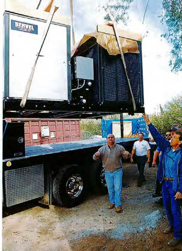
When the new chiller cooling system arrived, the plumbing and carpentry crews helped unload and install it. "Nobody ever said, 'That's not my job,'" says air-conditioning contractor Marshall Dennington.
