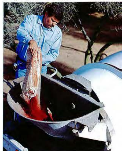
John Carson pours colorant in a concrete truck's hopper. It must churn for 30 minutes to ensure thorough mixing.
