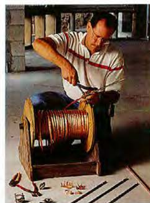
Installer David Vann clamps an air terminal to a length of copper cable.
