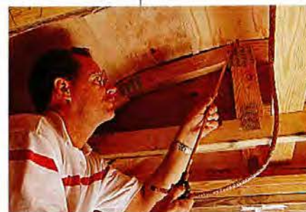
In the rafters, he identifies the spot where he will put the terminal through the roof.
