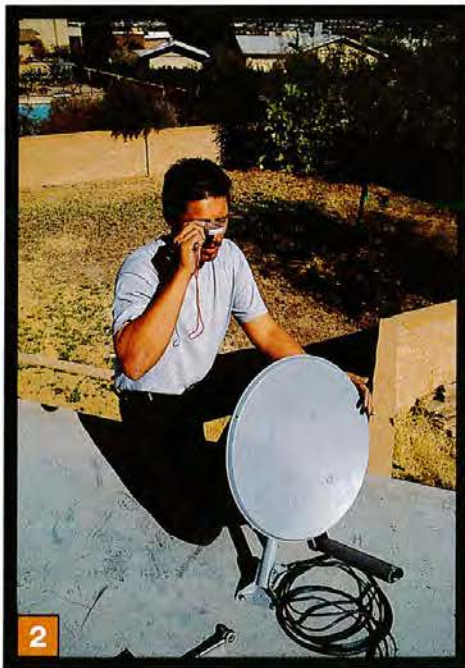
2 Using a compass, Camacho rotates the dish laterally to face its azimuth, the horizon point prescribed by the satellite service. Elevation is set with a built-in protractor behind the dish. Elevation and azimuth settings for every zip code in the country are programmed into the receiver.
