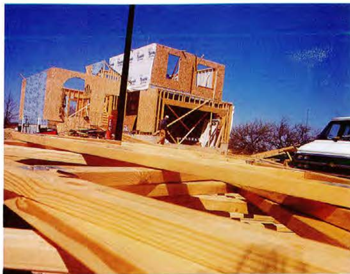
Trusses lay stacked and ready to be lifted by crane onto the roof of a newly framed tract house, one of the 1.35 million wood homes built every year in the United States. On average, 15,000 board feet of lumber is used in the construction of a single house.
