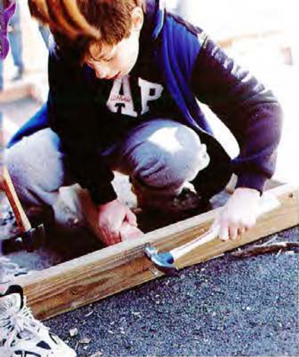
In framing a wall, 10-year-old Andrew Vitelli discovers it takes many whacks to drive a 3-inch nail.
