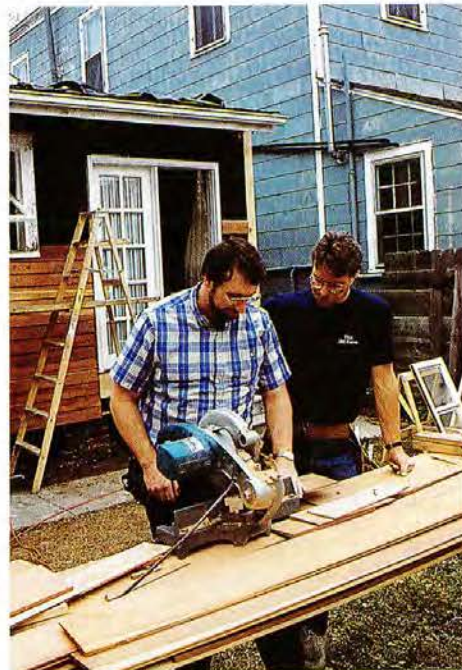
Norm and Steve get to work trimming clapboards for the rear of the twin houses.
