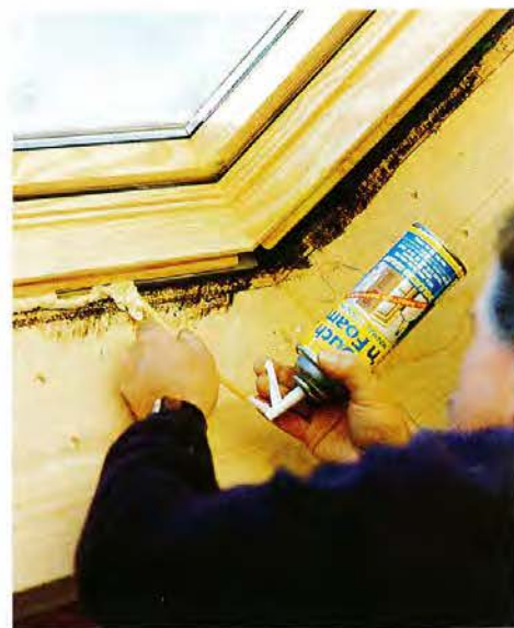
Urethane foam seals the gap between frame and skylight, preventing water from collecting on the flashing's underside. "A lot of people think their skylights are leaking," Tom says, "but they're really condensing on the inside."
