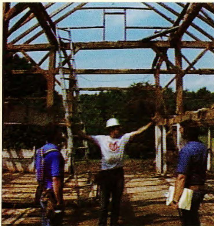
Framer Tedd Benson can read the history of a building in its timbers. After examining the original barn, he describes its construction to Steve Thomas, left, and Norm Abram.
