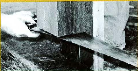
10" rotted bottoms of these load-bearing columns...
