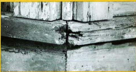
This rotted – and irreplaceable – woodwork...
