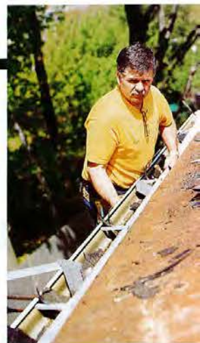
Dam fixer, p. 110
