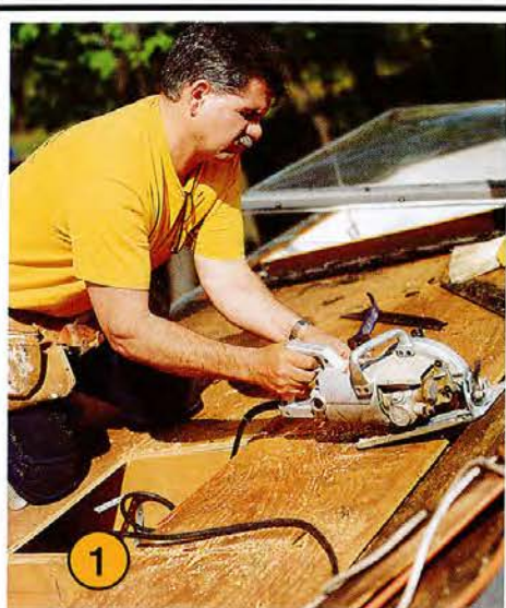
1 With the plywood sheathing exposed, Tom cut away portions to uncover trouble spots. Steve knew the flashing around the skylight leaked heat, but opening up the roof revealed more problems. Excessive amounts of heat also were escaping through recessed lights, a vent pipe and inadequate insulation.
