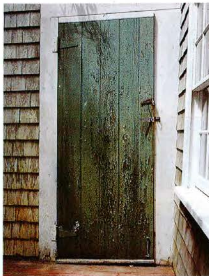
A batten door, on what's known as The Little Red House, is built like a ship's hatch.
