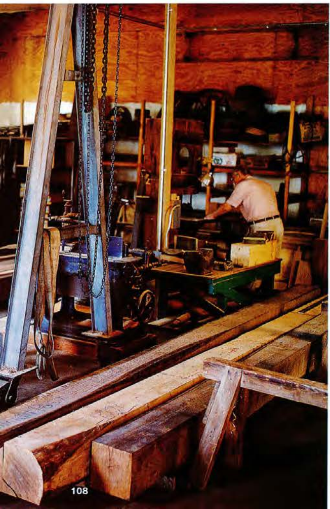
BELOW: Sixteen-foot beams will replace rotted wood in Burwell-Morgan's hurst frame, the giant table that holds all the mill's moving parts.
