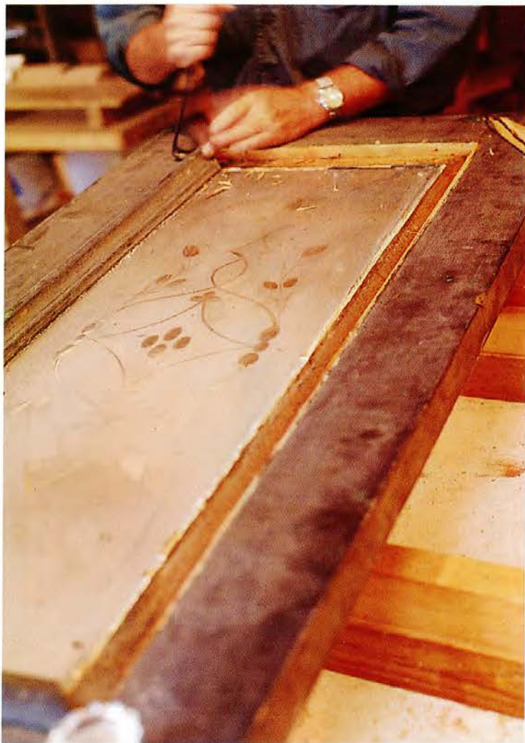
ABOVE: Tension is high in Bruce Killen's shop as moldings are pried off to free the surviving cut-glass pane. RIGHT: Cracks were filled with epoxy before the doors were cranked tight.
