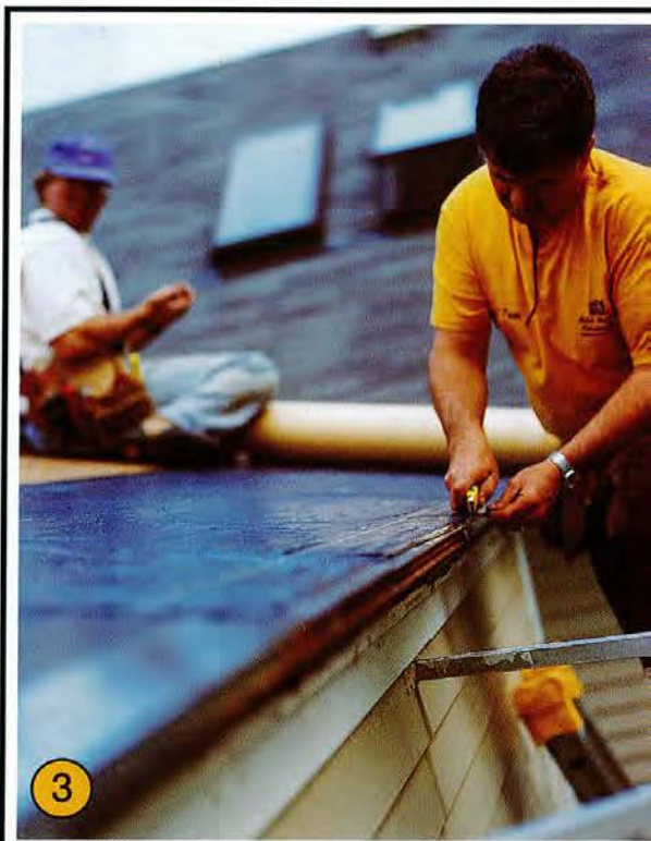
3 Installing the self-adhering membrane was “a little like tangling with a giant roll of flypaper,” says Tom. Two courses of this waterproof layer were laid in a 6-foot-wide strip along the eaves to protect the house from water that backs up behind an ice dam.
