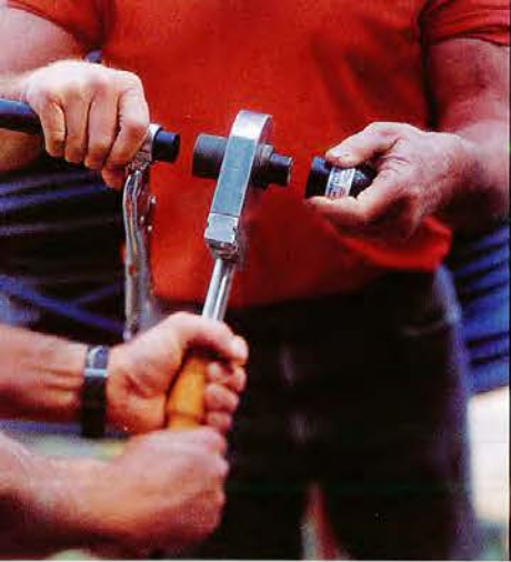
Each borehole contains two sections of pipe joined at the base with a hairpin coupling. The pipe is fused to the coupling using a 510-degree iron, creating a seal that won't leak.
