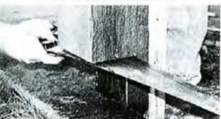
10" rotted bottoms of these load-bearing columns...
