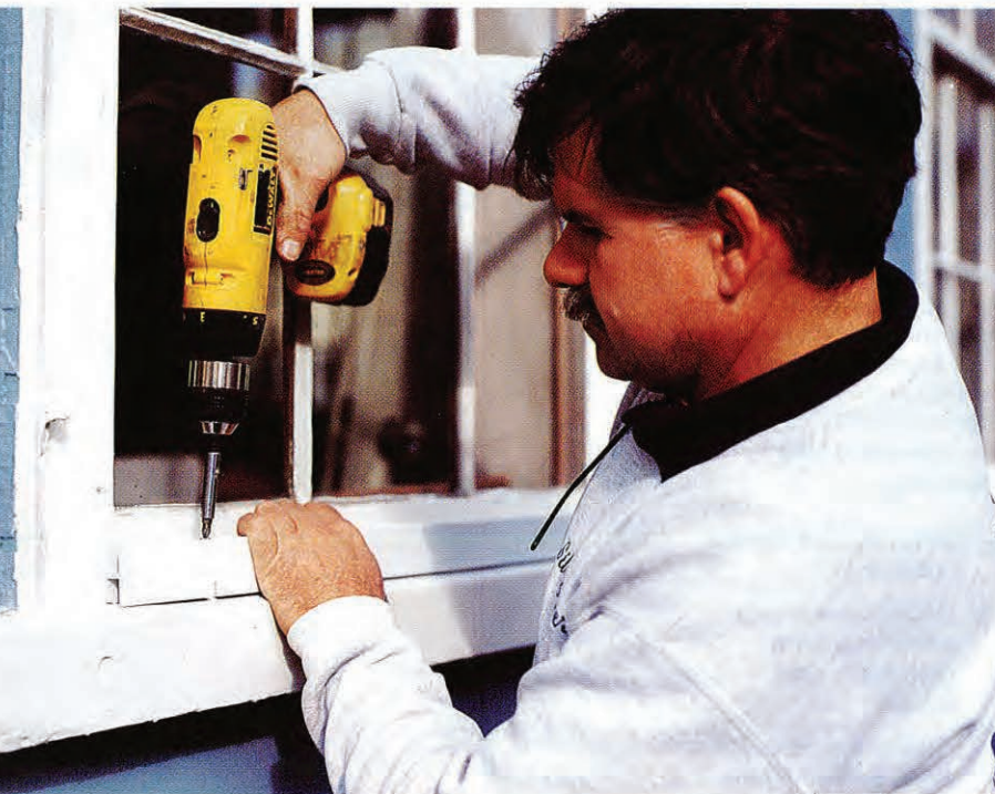
A cordless drill/driver is just right for installing storm windows. The switch on top is for changing speed ranges.
