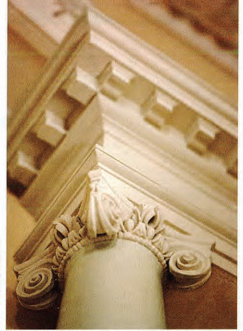
The Ionic capital and entablature of panel-molding cornice and modillions—all made of plaster—proclaim the Greek Revival influence at the Isaiah Davenport House, 324 East State Street (1815-20).
