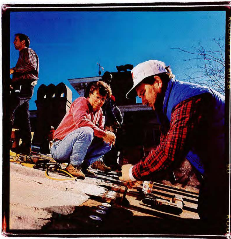
As Steve watches, roofing contractor Jeffrey Lancaster seals the seam between the new roof and the old.
