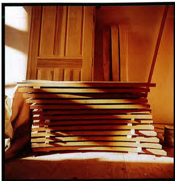
Neatly stacked stair treads wait for their introduction to the stringers. On this job, Lovely fabricated the treads in his shop and trucked them to the site, where they fit perfectly.
