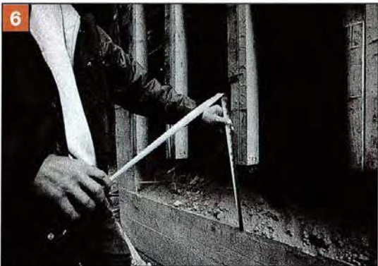
6 The first inches of the lift are the most crucial. All the connections that tie the house to the foundation should be severed before the procedure begins, but there are often spots that stick.
