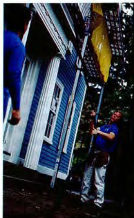
Setting up for the shoot is fairly simple, if a little strenuous: Heavy, high-pressure hoses that carry the materials have to be hauled up and fed in through a window.
