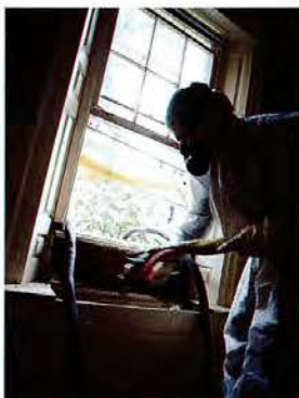
Built-in window seats at the Guinees' house are lovely details but also a big source of drafts and heat loss. With a few pulls of the trigger, Gustavo Nadasles plugs the leaks and fills the cavity. It's a case of giving up a little storage space and gaining big energy savings.
