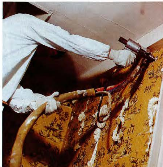
To fill a wall, Ted Franklin presses his gun into predrilled 1-inch holes. He starts at the midpoint and finishes near the top. Overflowing foam tells him the cavity is filled.
