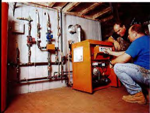
The two Richards, Trethewey and Bilo, ready the new microprocessor-controlled boiler for three functions: warm air, warm floors and hot water.
