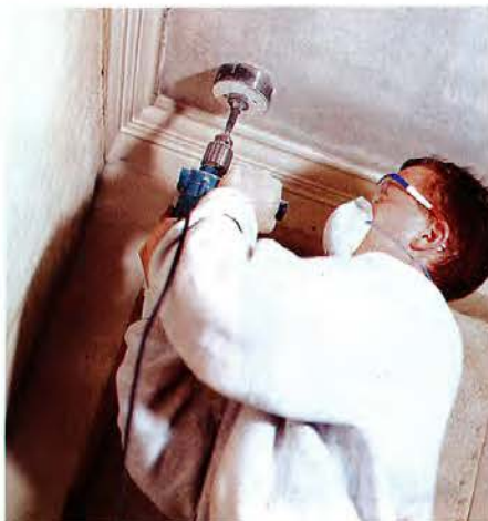
To bring a warm air outlet into a room, Brian Bilo starts by drilling a 4-inch hole through the plaster and lath in the ceiling.
