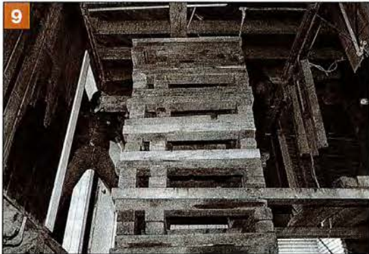
The stack of cribbing grows as the house rises. The house remains on the cribbing for two months while a new foundation is poured and wooden piers are set. Then A.C. Hanna returns and lowers the structure onto the new foundation.
