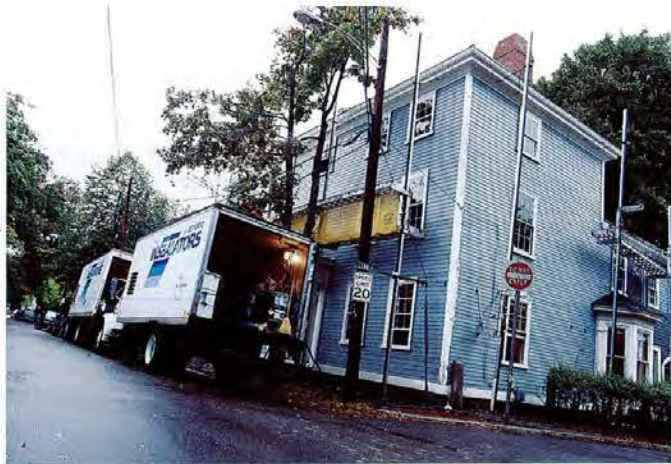
LEFT: Insulation day at the Guinees'. The chemicals and machinery stay on the trucks; only the spray hoses go inside. BELOW: Richard Trethewey and heating contractors Richard and Brian Bilo wrangle the new boiler into the basement.
