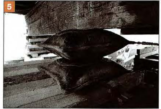
Because of the size of the Coen house, the jacks were augmented with air bags. The jacks and air bags must be synchronized to move at exactly the same pace. If one jack or airbag is off by as little as an inch, the house will pitch and corkscrew.
