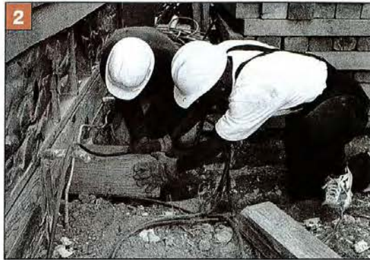
2 Holes are jackhammered in the foundation wall so that 8-by-8-inch timbers can be slid under the house, perpendicular to the floor joists, to support the structure as it begins its upward climb.
