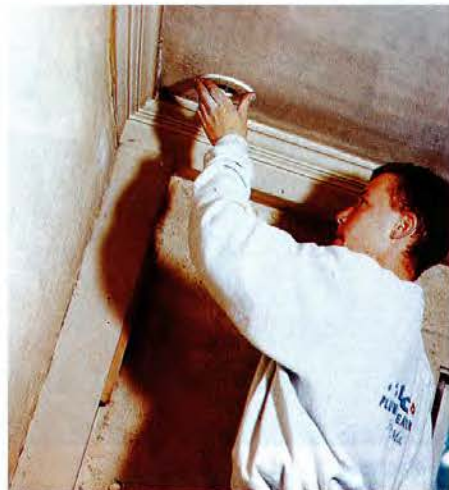
When the job is finished and the outlet is in place, it's barely noticeable. The plastic can also be painted to further camouflage it.
