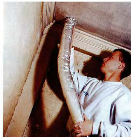
With a helper pulling from above, he feeds the duct up into the attic. If needed, additional lengths can be coupled on up there.
