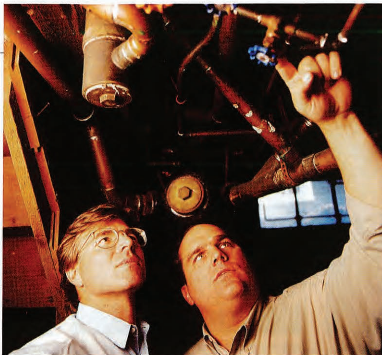
This, Richard tells Steve, is a plumbing nightmare: a jumble of unsupported pipes made of several different materials, arranged in patterns that appear to defy logic.
