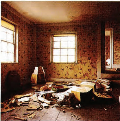
Stains in ceilings, Sutton says, are a red flag to check for a leaking roof.
