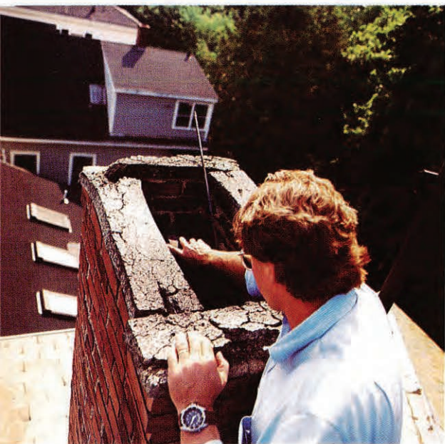
Steve checks loose and crumbling mortar work atop a chimney on the oldest part of the house.
