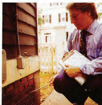
Brick is not an ideal foundation material, and on the Victorian addition it needs to be repointed.
