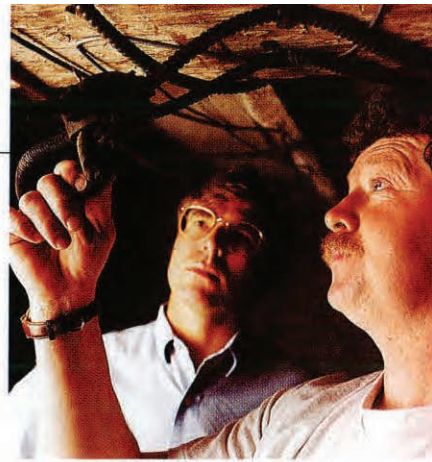
Steve and Paul test the soldered connections in a basement junction box.
