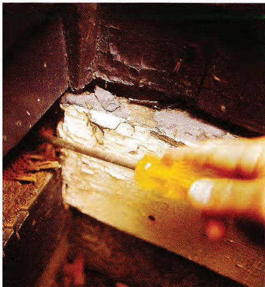
Obvious rot in trim and siding usually signals even more extensive trouble inside the wall.
