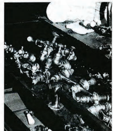
Faucets and components line the walls of the plumbing room.
