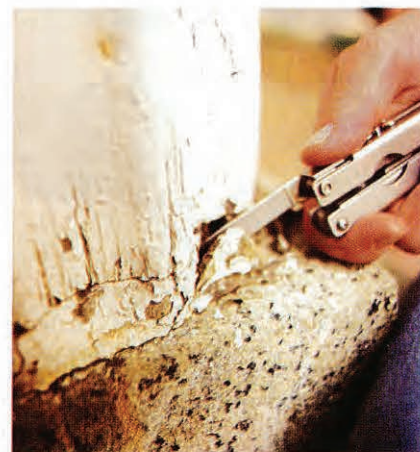
Steve's Multi-Plier detects rot at the base of a column on the front porch.
