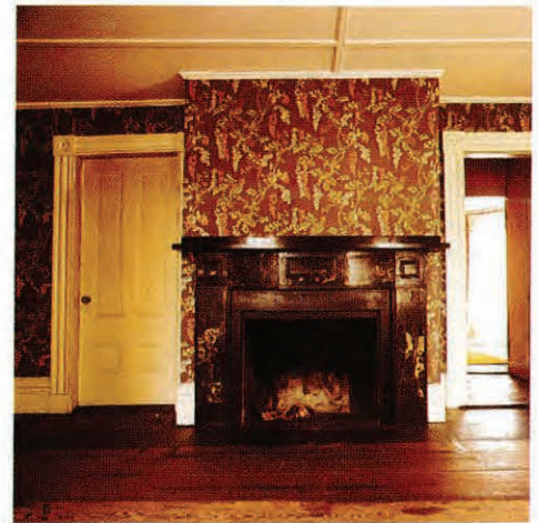
Sagging door frames next to a fireplace indicate uneven settling problems.
