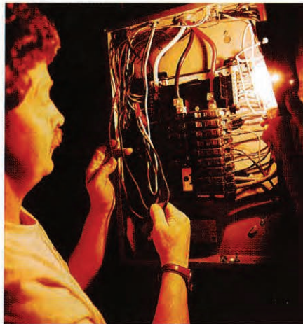
The main circuit-breaker box is the first stop on a thorough examination of home electrics.
