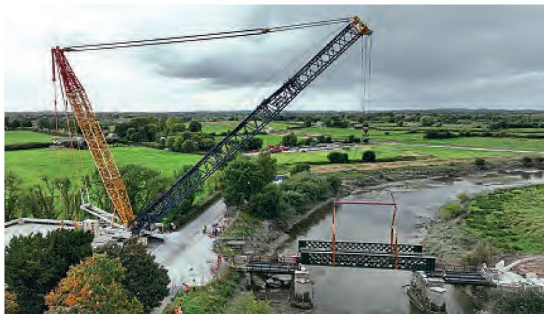
Ireland's largest crane was assembled on site at Adare to lift the refurbished centre span back into place on September 24. This was the last structure needed to be completed before track laying can continue to Limerick. IARNRÓD ÉIREANN
