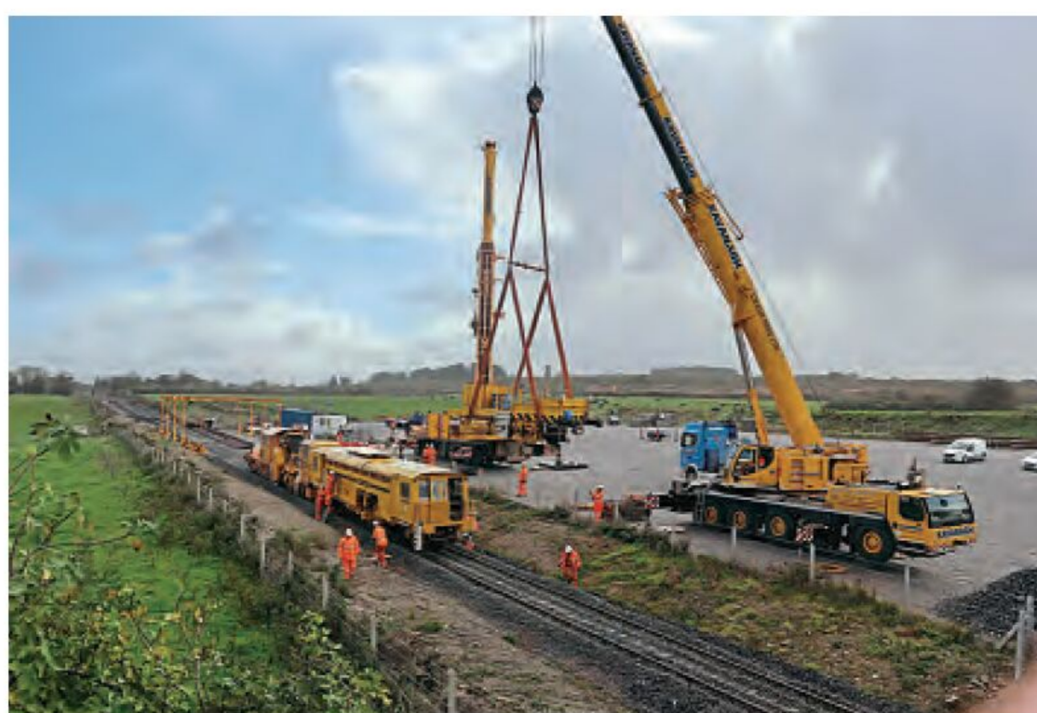
Iarnród Éireann tamper No. 742 and ballast regulator No. 704 were delivered from Limerick Junction by road to the compound at Glenbane East, near Foynes on October 17. This will allow the line track to be aligned and tamped in readiness for the lines reopening in early 2026. The Tamper and Regulator operated by Rhomberg Sersa is expected to be on site for at least six months. TREV BEACOM
