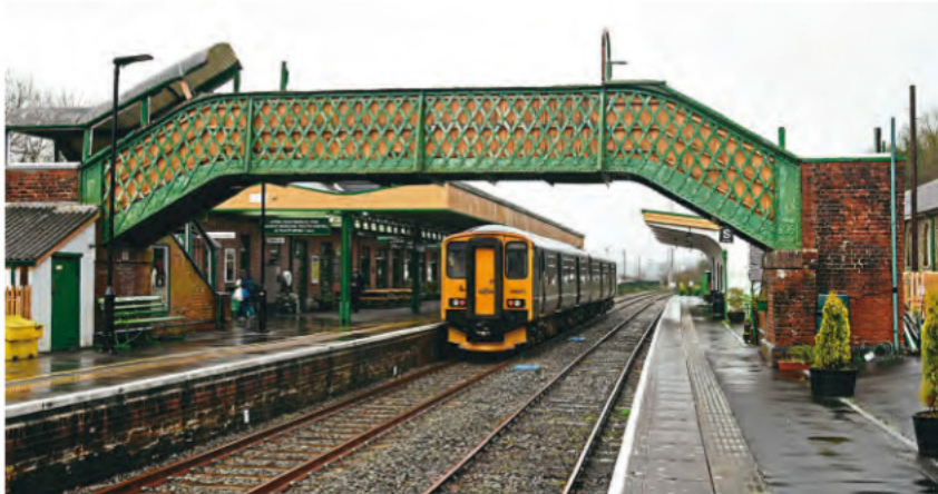
LEFT: One of this winter's series of storms, Storm Henk, blew the roof off the footbridge at Okehampton station around midday on January 2, 2024 as No. 150247 was on the branch with the 11.32 from Exeter Central. The DMU was stopped before reaching the station and given permission to proceed to the east end of the platform so that passengers could exit via the front set of doors. The service was then cancelled until the following day, when No. 150221 is pictured under the damaged footbridge with the 14.26 to Exeter Central. D W V HUNT
