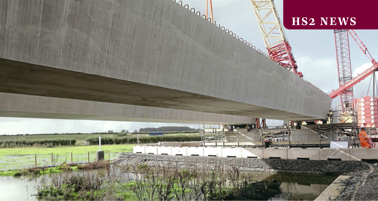
Two of the 72 beams in position, showing the height of the Thame Valley viaduct over the river's floodplain. ALL PHOTOS TAKEN ON OCTOBER 30 BY PHIL MARSH
