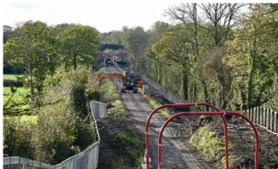
Work continues on refencing and clearing the Foynes line of all vegetation within the railway boundary. With all track now removed, Sisk contractors are seen at Clonshire, near Adare, preparing the trackbed for the installation of the signalling and cabling ducts and track laying. The wooden fencing to the right is horse fencing and the orange flexi piping is for diverting the fibre optic cable which was laid in the line in the late 1990s. Track laying is due to start in January. HASSARD STACPOOLE
