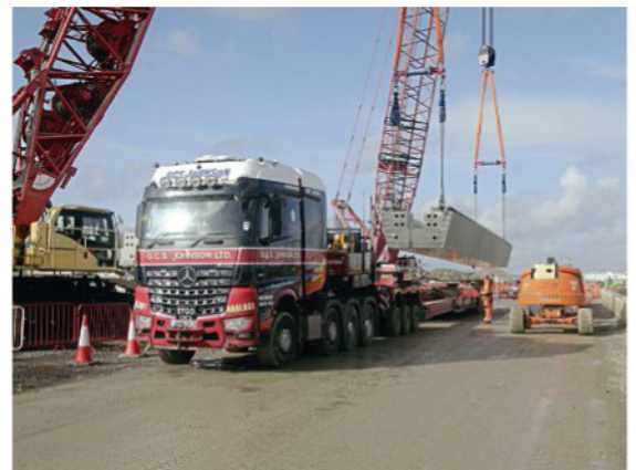
A 90 tonne beam arrives by road from the factory on the Isle of Grain.
