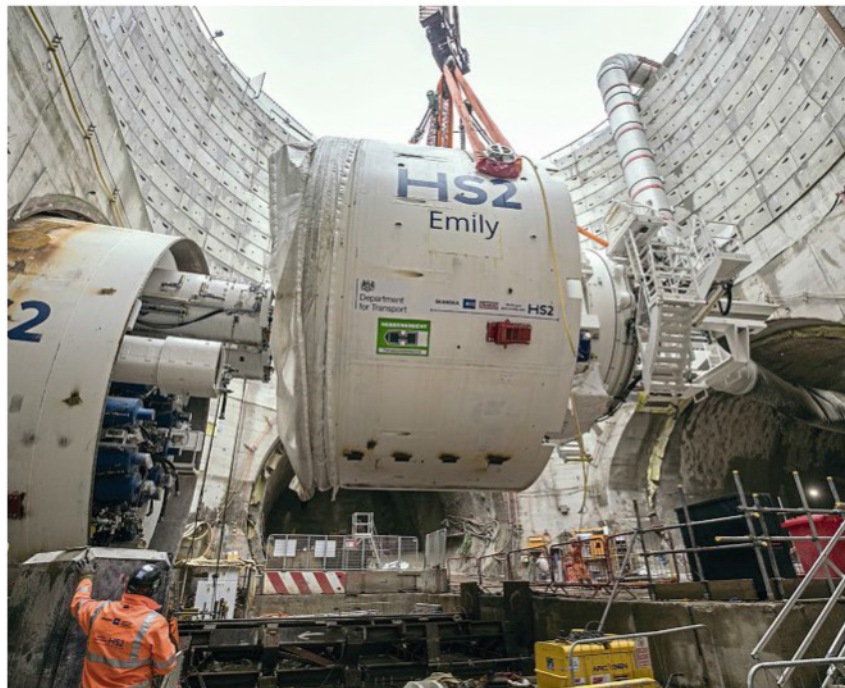
weigh 1700 tonnes and have eight back gantries each, carrying all the systems required for the tunnelling operation.
