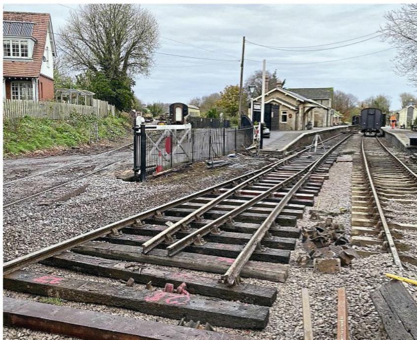
Track work in progress at the East Somerset Railway's Cranmore station on November 20. ESR
