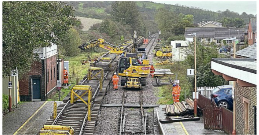
Almost half of CP7 spending will be on track, signalling and structures renewals. This is upgrade work at the south end of Maiden Newton station, Dorset, in October. NETWORK RAIL
