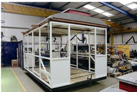
One of the cars being refurbished at Wheel Sets UK in Rotherham on June 23.
