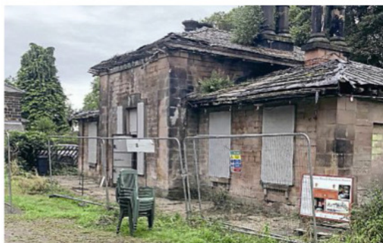
With trees growing in the roof, this was the sorry state of Wingfield station prior to restoration commencing in 2019. DHBT
