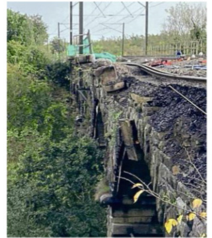
Plessey Viaduct's north-eastern corner showing the extent of the parapet repairs being undertaken. Network Rail
