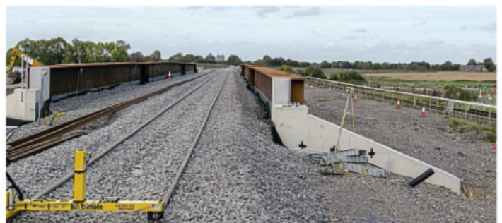
A view north along the bridge showing its design can accommodate a second track. The old line, which will be severed by the HS2 excavations, is on the right. BOTH: CHRIS MILNER
