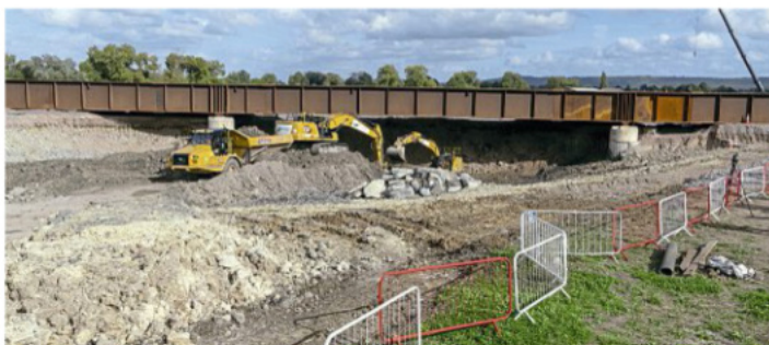
Work to remove thousands of tons of earth from underneath the new bridge on the Aylesbury-Princes Risborough line in order to create the trackbed trace for HS2.
