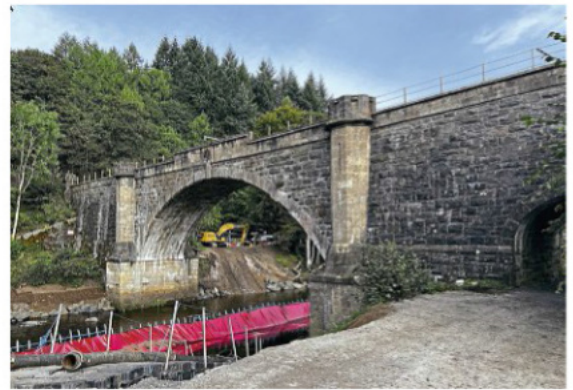
Inver viaduct at Dunkeld with scour protection work taking place. NETWORK RAIL
