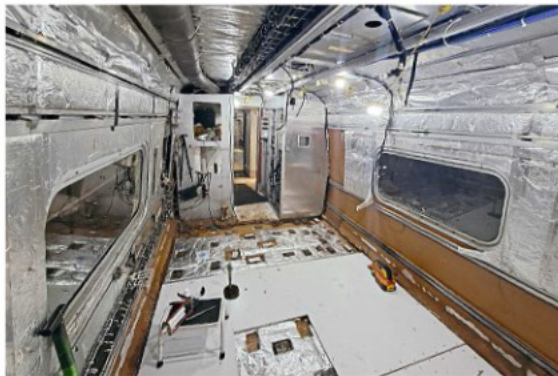
Inside one of the stripped-out carriages of No. 390050. Hard to believe it would be back in traffic just 10 days later.
