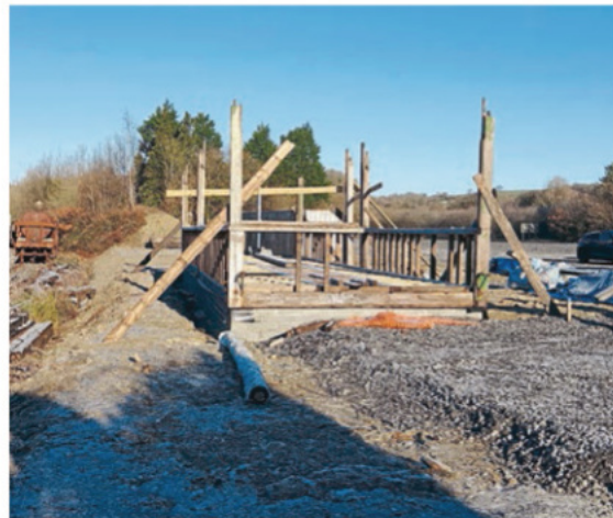
Swansea Kings Dock Junction signalbox is being rebuilt as the office and shop at Abergwili Junction station. The current platform, running line and loop are on the left. A future plan is to build a second platform alongside the loop for easier public access to the trains. The car park is to the right. DEWI JONES
