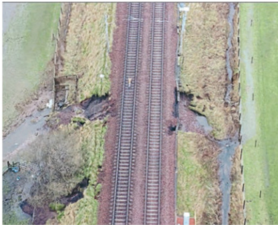
The damage seen from the air on December 31. NETWORK RAIL
