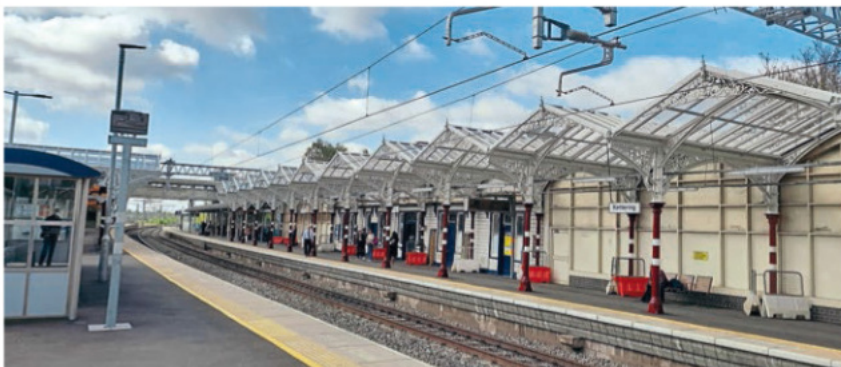
Kettering station's platform 4 with its restored and cleaned Midland Railway canopies. NETWORK RAIL
