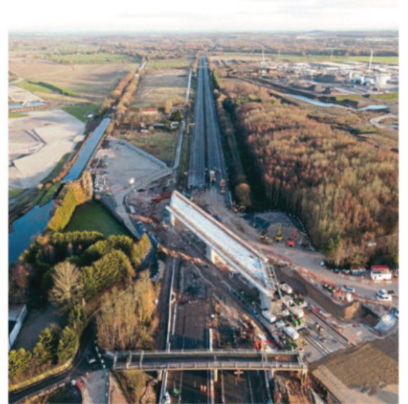
The bridge is pictured in the process of being positioned over the M42 at Lea Marston, near Kingsbury in Warwickshire. HS2
