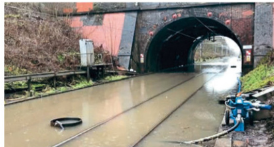
NR is expected to plan for the effects of climate change and extreme weather to help avoid events such as this flooding at Culcheth, north-east of Warrington, due to Storm Christoph in January 2021. NR
