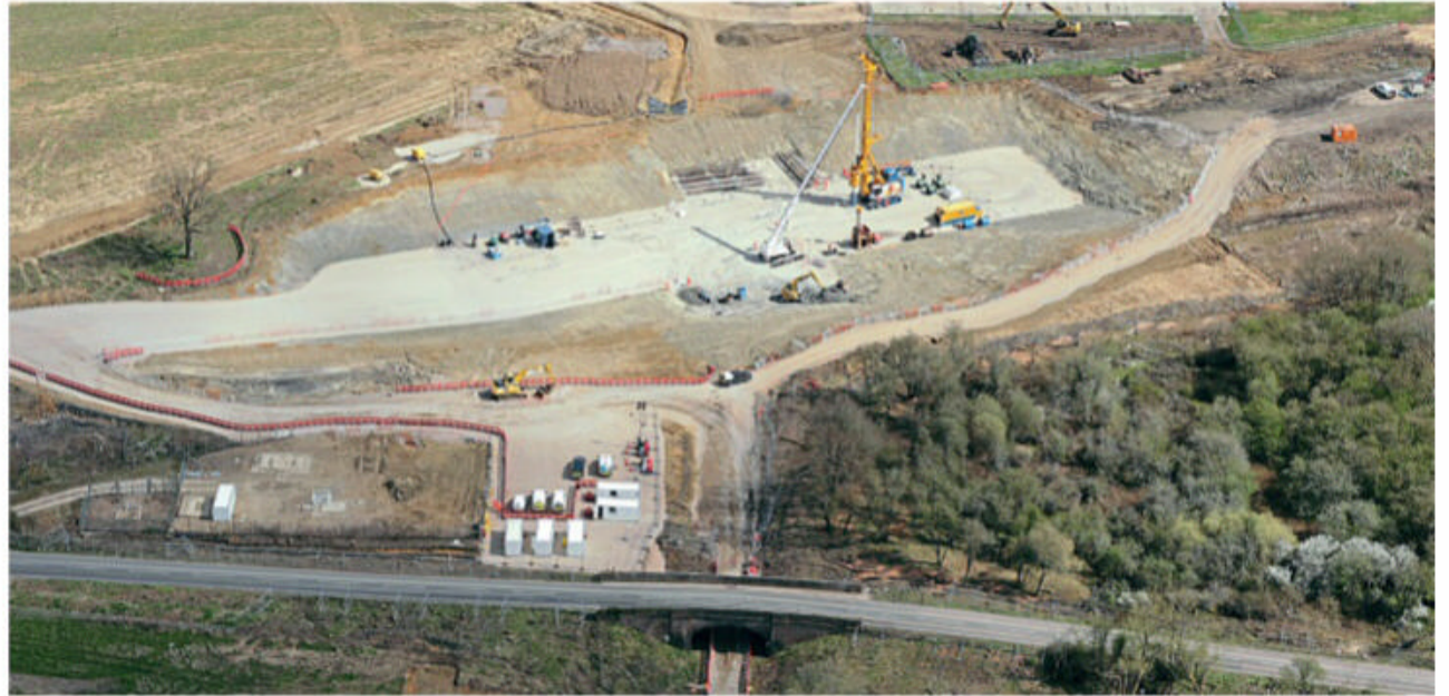
Looking east at the Calvert worksite in Buckinghamshire where HS2 (running right to left) will pass under East West Rail.
