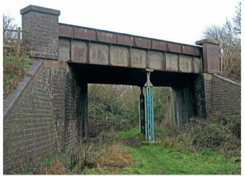
The support under the bridge at Collin Lane in Willersey, north of Broadway. The Gloucestershire Warwickshire Railway is working to ensure the bridge does not get filled in. JO ROESEN
