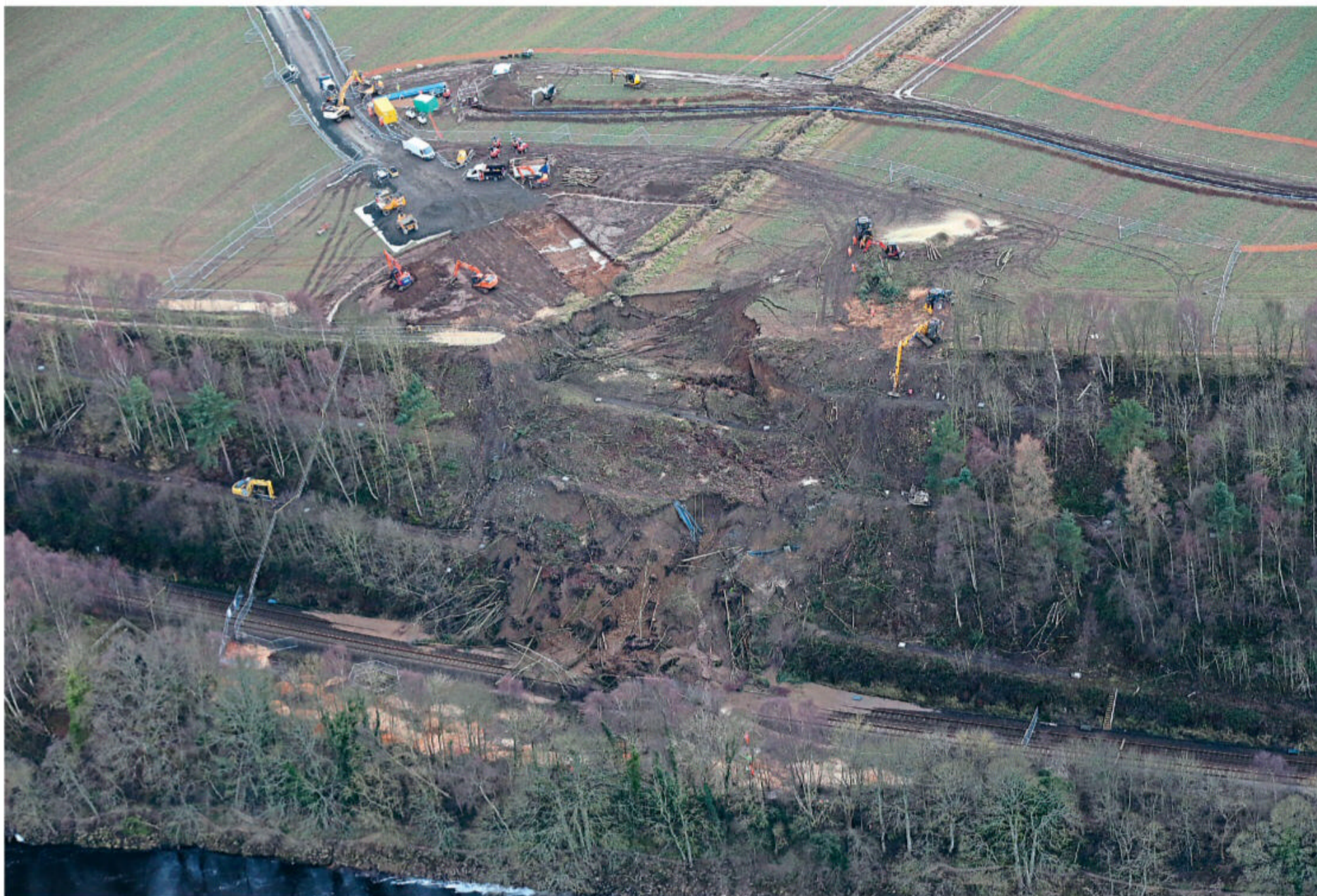
One of the advantages of using helicopters is in getting an overall view of events like this one near Hexham on January 14, 2016, where flooding has caused the cutting to collapse onto the running lines.
