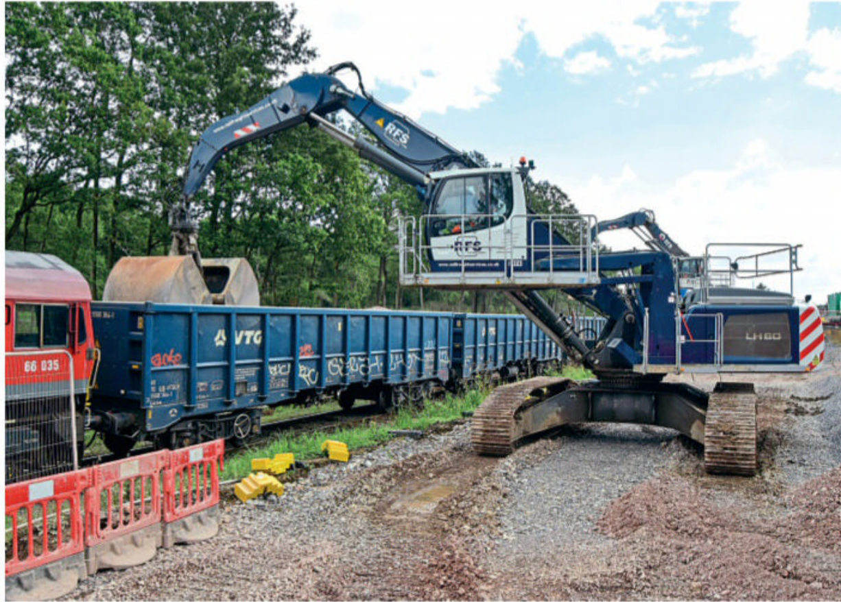
Excavators prepare to transfer aggregate from a train hauled by Class 66 No. 66035 at Calvert South to dumper trucks for stockpiling ahead of use in the HS2 construction project. HS2
