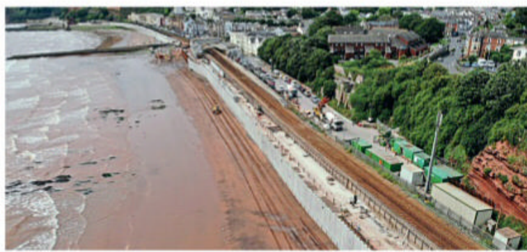
Work on the sea wall panels taking place between Dawlish station northwards towards Rockstone Bridge. NETWORK RAIL
