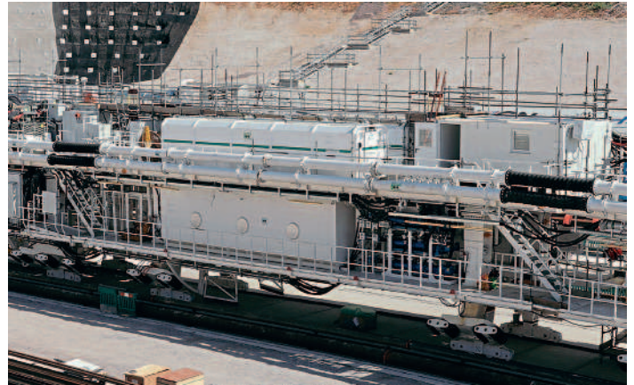
Cecilia's emergency refuge pod in Gantry 6, which is marked with a green line.
