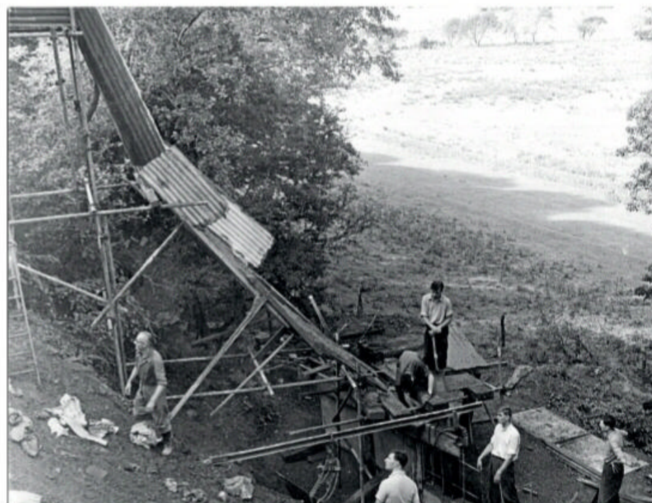
A chute made of scaffolding, corrugated tin sheet and wood for tipping concrete to create a retaining wall at the bottom of the Dolgoch landslip. TR ARCHIVES
