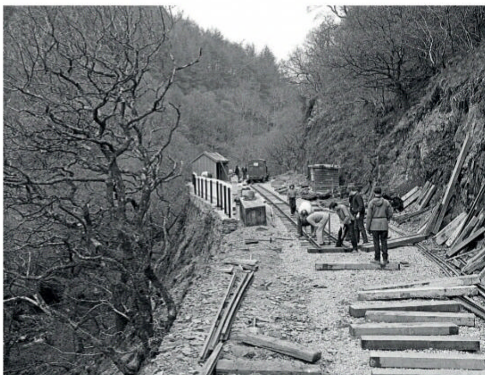
Laying the track out of Nant Gwernol station for the extension. The perilous drop off the edge along which the track originally ran can be seen on the left.
