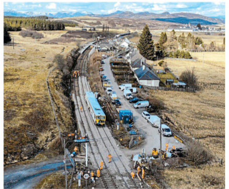
A drone view of the plain trackwork installed to get the line reopened. NETWORK RAIL
