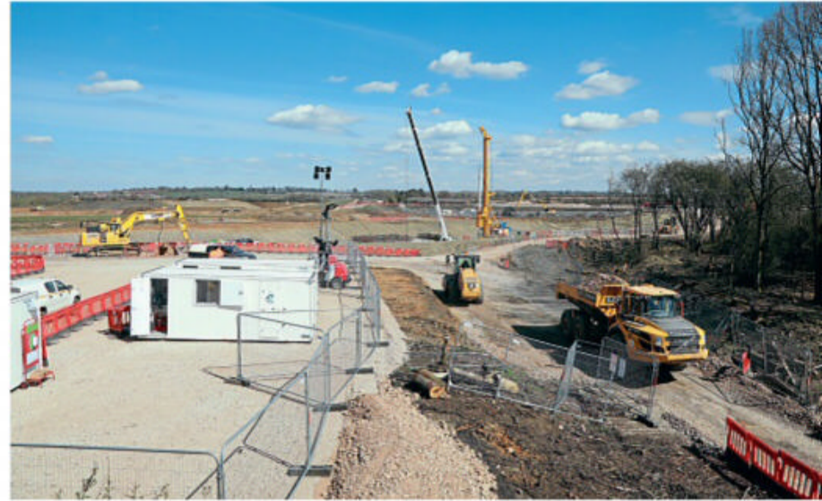
Construction work is underway on the bridge that will carry East West Rail over HS2 at Calvert in Buckinghamshire. HS2 contractors are building three bridges and around 3km of earthworks on behalf of EWR. PHIL MARSH
