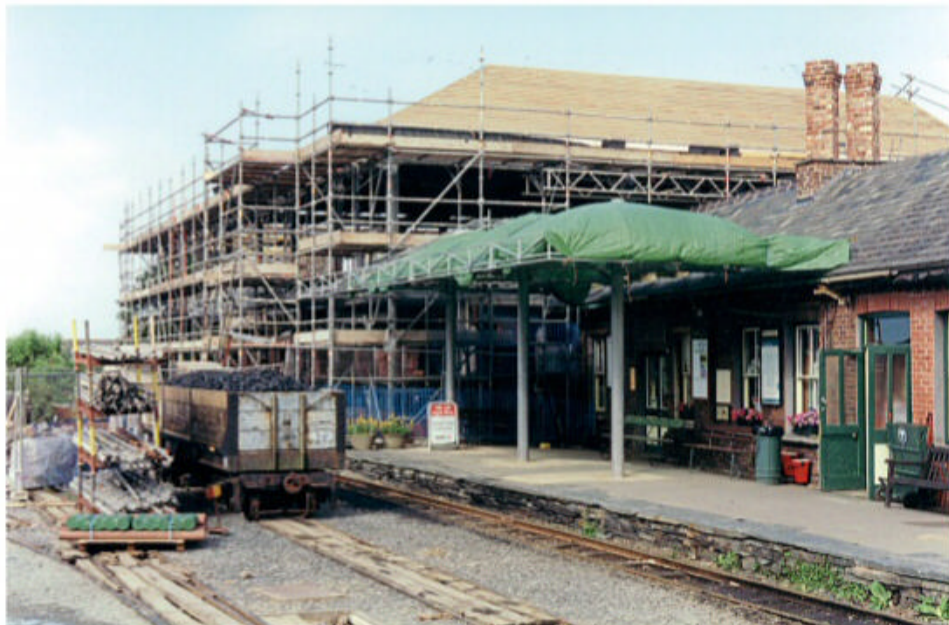
Wharf station was substantially redeveloped and expanded from the simple building inherited in 1951. Pictured in 2004, this view shows work in progress. DAVID MITCHELL
