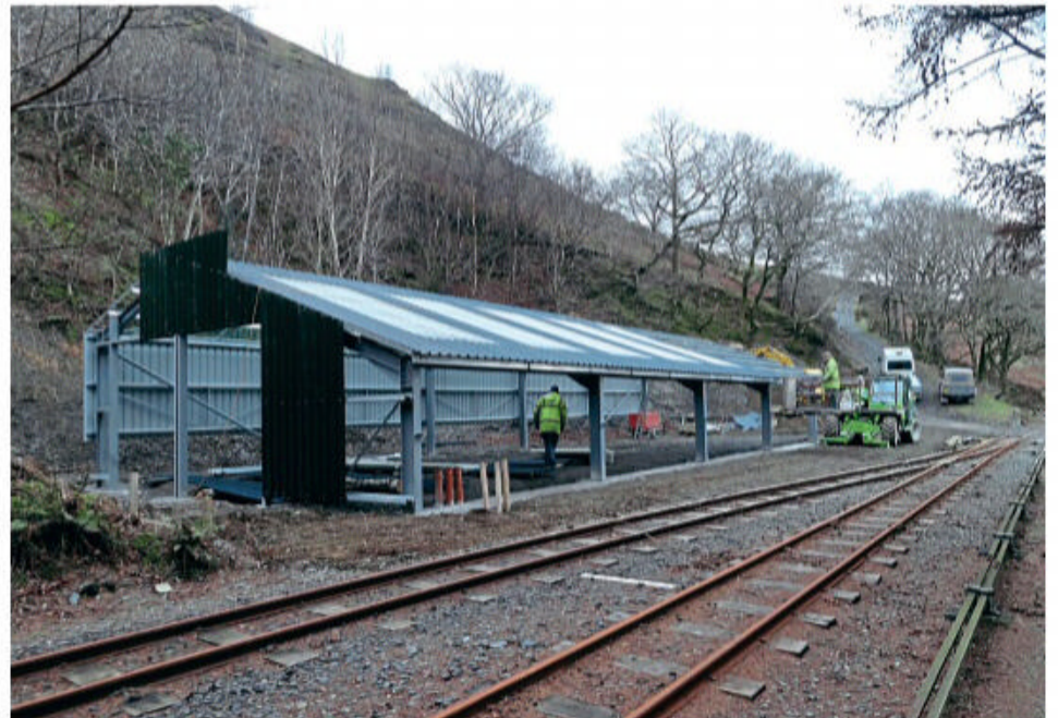
Construction of a new carriage shed during 2012, located five miles up from Tywyn at the site of the former Quarry Siding. It is named The Guest House, after Phil Guest, a long-serving Talyllyn volunteer, and was formally opened on May 5, 2012, by long-time supporters of the railway, Timothy West and Prunella Scales. KEITH THEOBOLD
