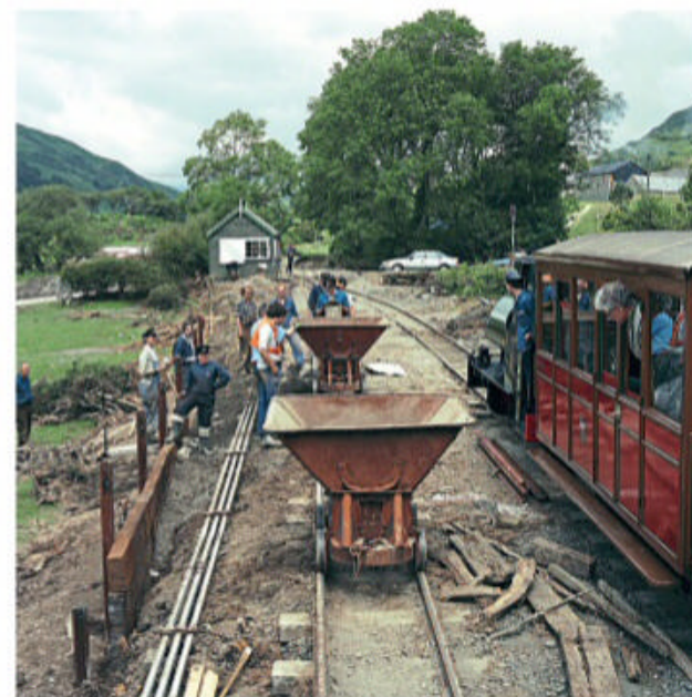
A work gang pauses during the task of filling tipper wagons at Brynglas, repairing flood damage as the up train passes.
