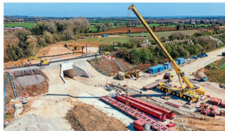
Although much of the engineering work undertaken over the Easter holiday was focused on the West Coast Main Line, the Chiltern Main Line was also closed at Bicester to allow a new underbridge to be slid into place. NETWORK RAIL
