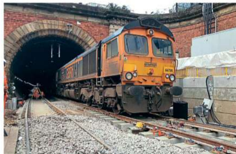
On March 6, GBRf's No. 66726 Sheffield Wednesday became the first locomotive to work a train through the eastern bore of Gasworks Tunnel since 1977. JOANNA THOMAS/NETWORK RAIL
