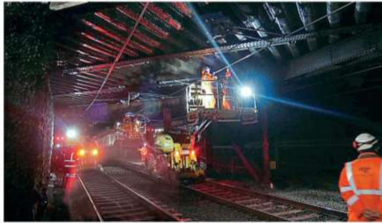
Network Rail engineers applying insulating paint to the underside of Intersection Bridge in Cardiff. JOHN SHERIDAN
