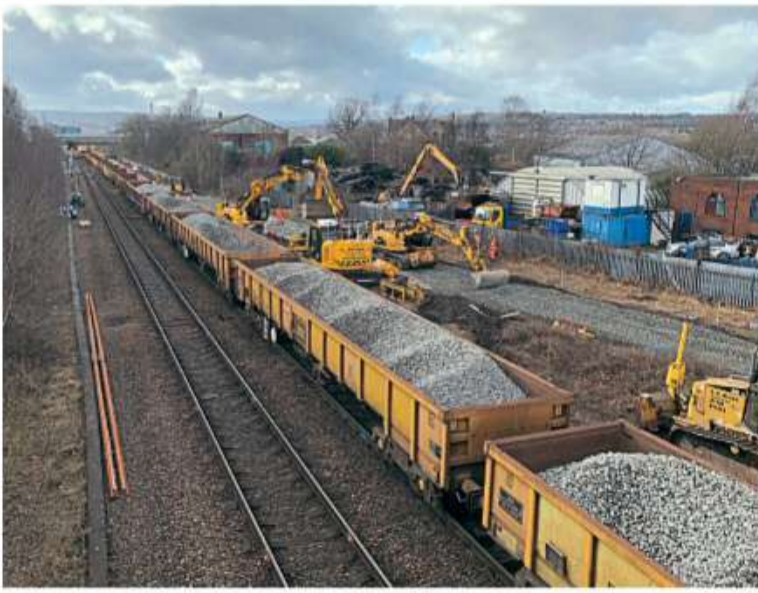
Track replacement work on the former Great Central Main Line at Woodburn Junction, Sheffield, on March 13. JOHN SHERIDAN
