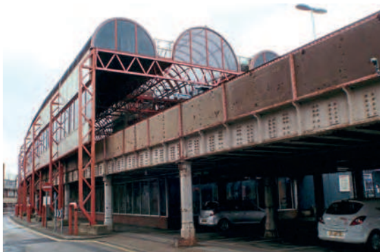
Services to Portsmouth will be disrupted in January as Network Rail closes Landport Viaduct for repairs. The Victorian structure carries the elevated line to Portsmouth Harbour through the heart of the Hampshire city. NETWORK RAIL
