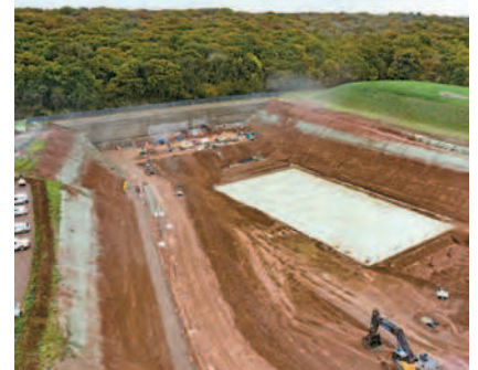
Preparation of the site to bore Long Itchington Wood Tunnel's north portal. BOTH: HS2.
