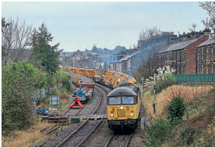
Engineering works between Harrogate and York in late-November brought the rare sight of locomotives to the North Yorkshire spa town. On November 28, Colas Railfreight No. 56087 powers past Dragon Terrace with a train of Network Rail switch and crossing carriers. CHRIS GEE
