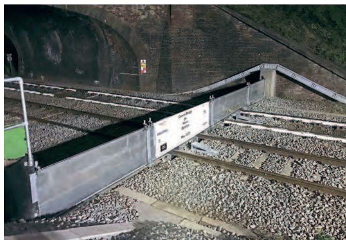
Right: Cowley Bridge, near Exeter, has suffered from flooding for many years. As well as huge investment in better drainage, Network Rail has taken the unusual step of installing temporary flood defence barriers to protect the railway. NETWORK RAIL
