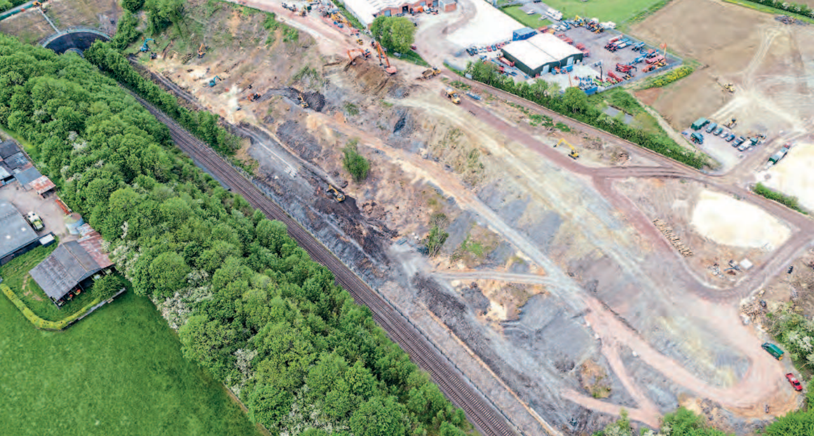
Heavy and prolonged rain can weaken earthworks, many of which are now more than 150 years old and have inadequate drainage for modern requirements. Unstable embankments and cuttings present a major safety risk and repairs often require extensive civil engineering works, as was the case at Harbury Tunnel, near Warwick, in 2019. NETWORK RAIL
