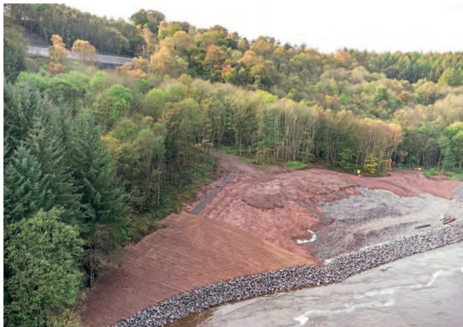
Overflowing rivers can scour away material, weakening embankments and bridge supports, creating safety risks for the railway. This aerial view of the repairs at Eden Brows on the Settle to Carlisle Line shows the extent of the work that was necessary to shore up the huge embankment after heavy rains in 2016. NETWORK RAIL
