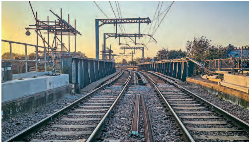
Repairs have been completed to track and timber bridge supports on the largely elevated Gospel Oak to Barking line in north London. More than two miles of track and supporting timbers on several bridges were damaged by a derailed freight wagon in January 2020. NETWORK RAIL
