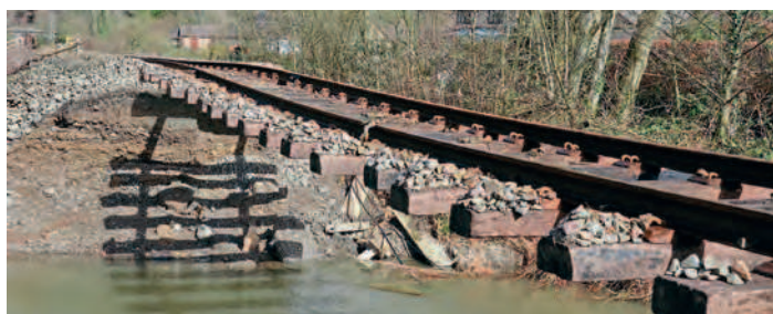
Above: The Conwy Valley Line in North Wales has suffered two prolonged closures in the last three years as a result of flash floods washing out the track around Dolgarrog and Llanrwst. NETWORK RAIL
