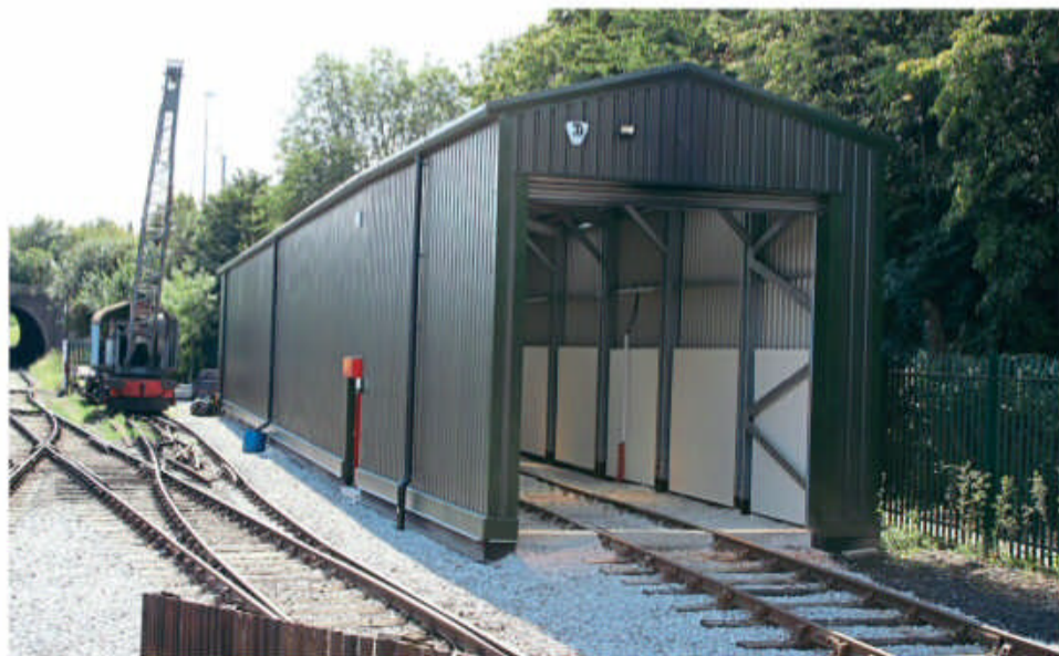
Vandalism and arson has plagued the railway, but the line's recently constructed carriage shed is designed to protect rolling stock from further damage. OLIVER EDWARDS
