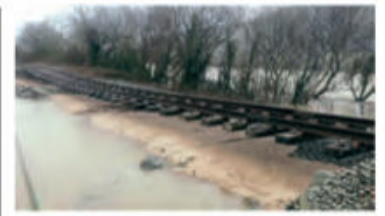
Track washed out from the floods in February this year as a result of Storm Ciara. The damage was not as substantial as from 2019's Storm Gareth, which closed the line for four months. NETWORK RAIL
