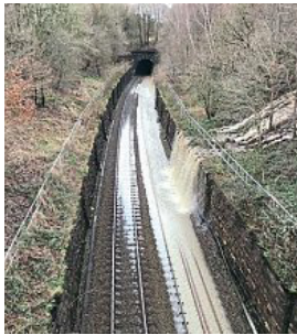
Water cascades onto the track at Bramhope Tunnel.
