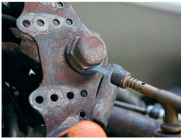
Heat was required - and worked
