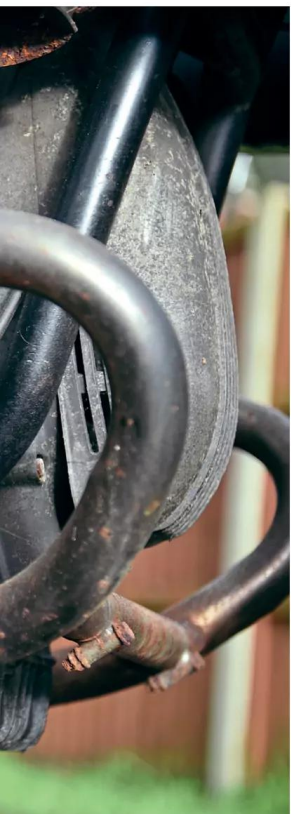
Right: Master cylinder is under the tank and looks bad
