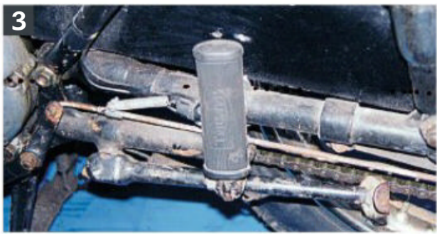
3: This shot shows the true nature of the beast and how much work will be required to get this lot looking like new.
