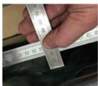
The dent at its deepest point was 20mm, causing distortion elsewhere
